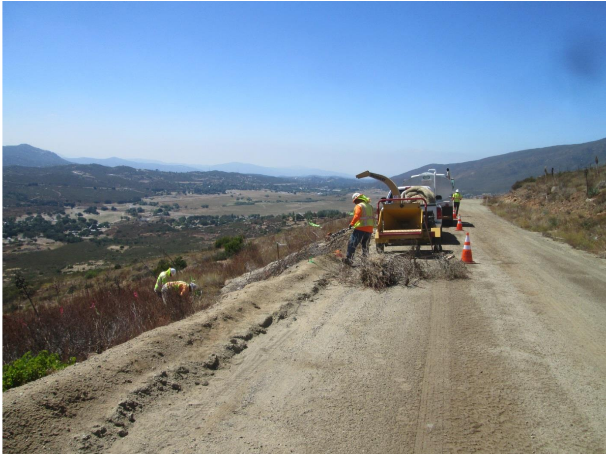
Photo 3: Vegetation clearing activities observed along C78. Traffic control notification signage, cones, and flagpersons were observed along Viejas Grade Road in accordance with APM TRANS-02.
