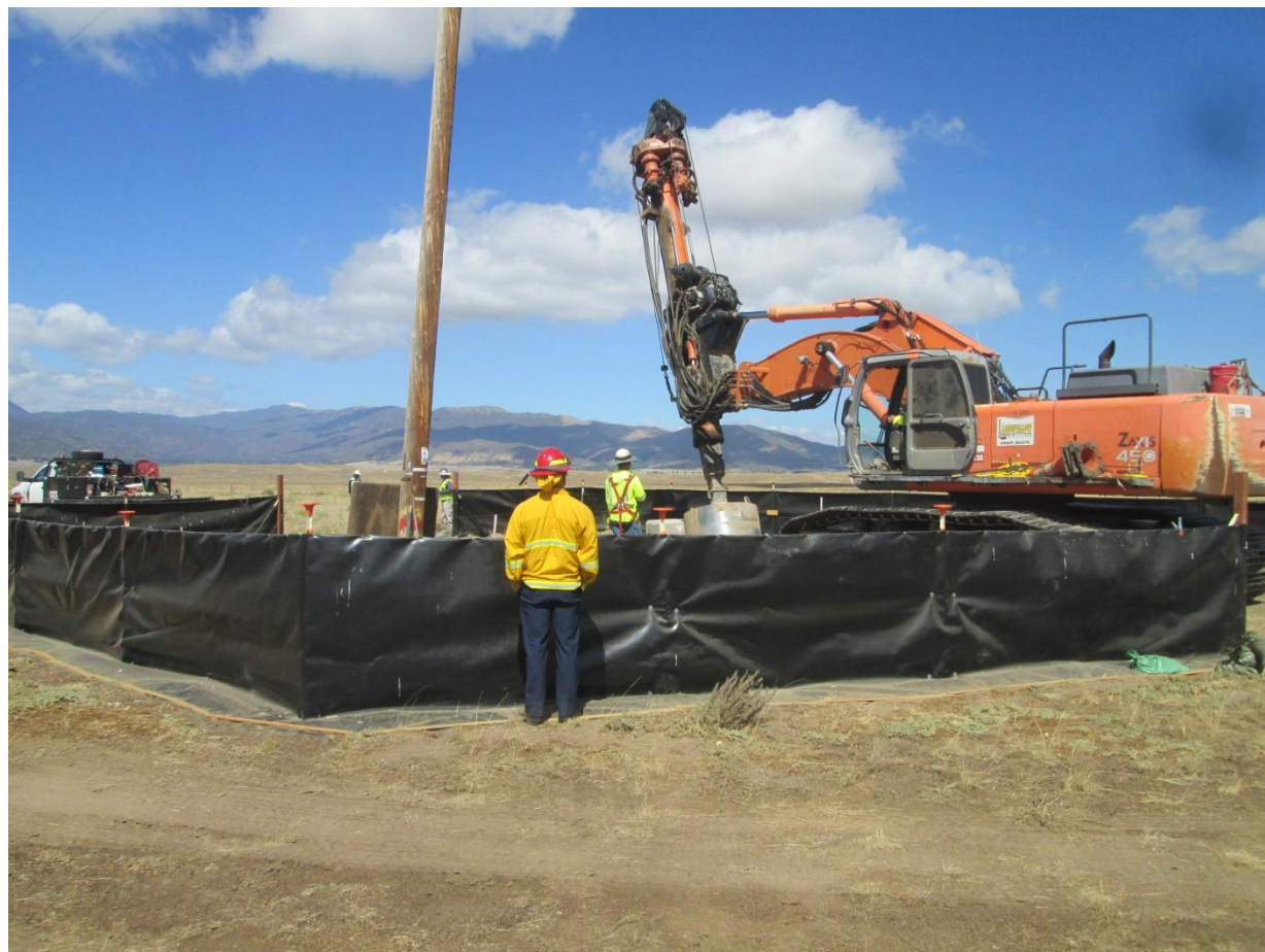
Photo 2: Pole hole drilling observed at Pole Z118221 (TL 682) within Stephens' kangaroo rat exclusion barrier (MM BIO-31). A fire patrol was observed monitoring construction activities in accordance with the Construction Fire Prevention/Protection Plan (MM FF-1, APM HAZ-1).
