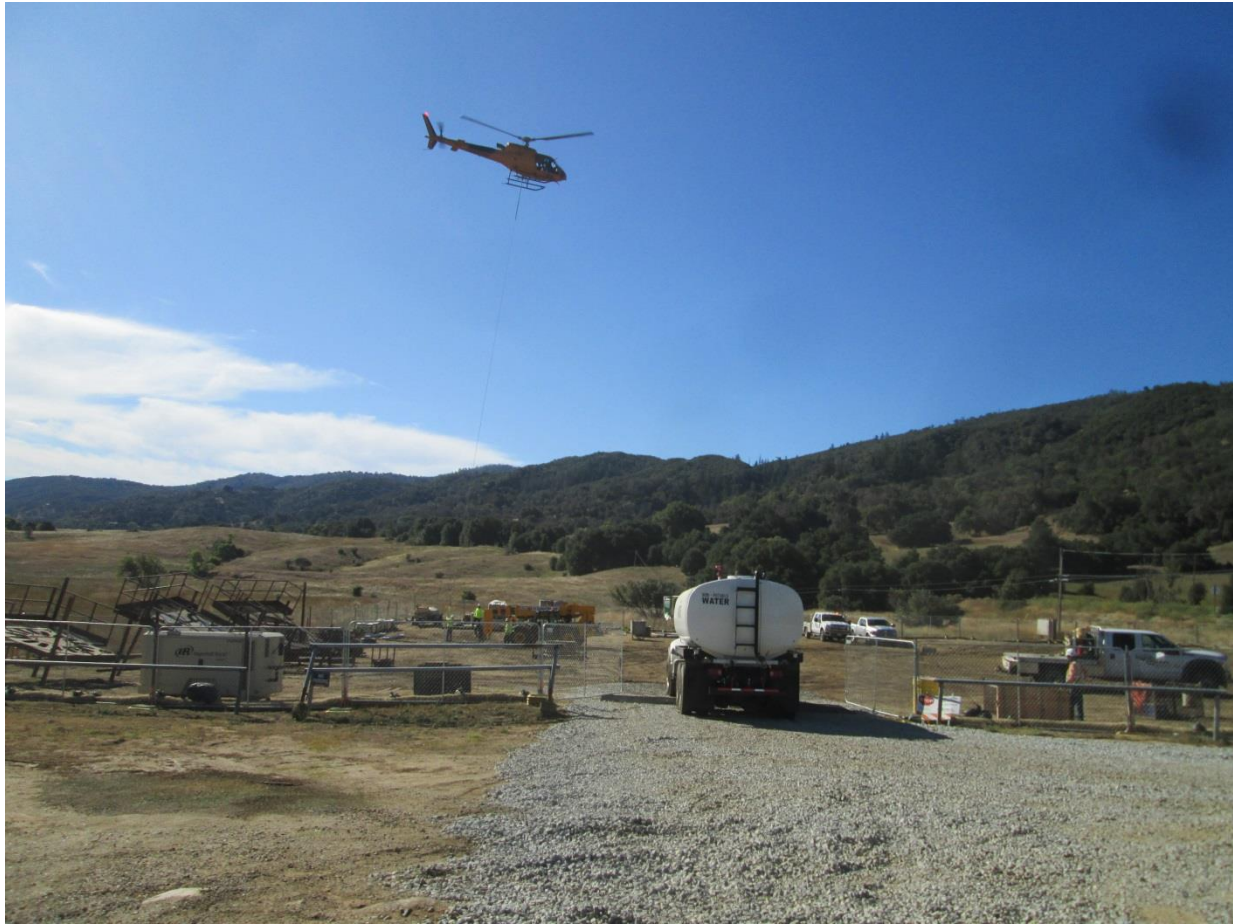
Photo 4: Helicopter external load operations were observed being conducted out of Lake Henshaw Staging Yard (TL 682) to assist foundation drilling and grouting operations at remote site along the project alignment. To prevent potential dust emissions from rotor wash in accordance with the Aviation Safety Plan (MM PHS-5), a water truck was utilized to apply water within the work area.
