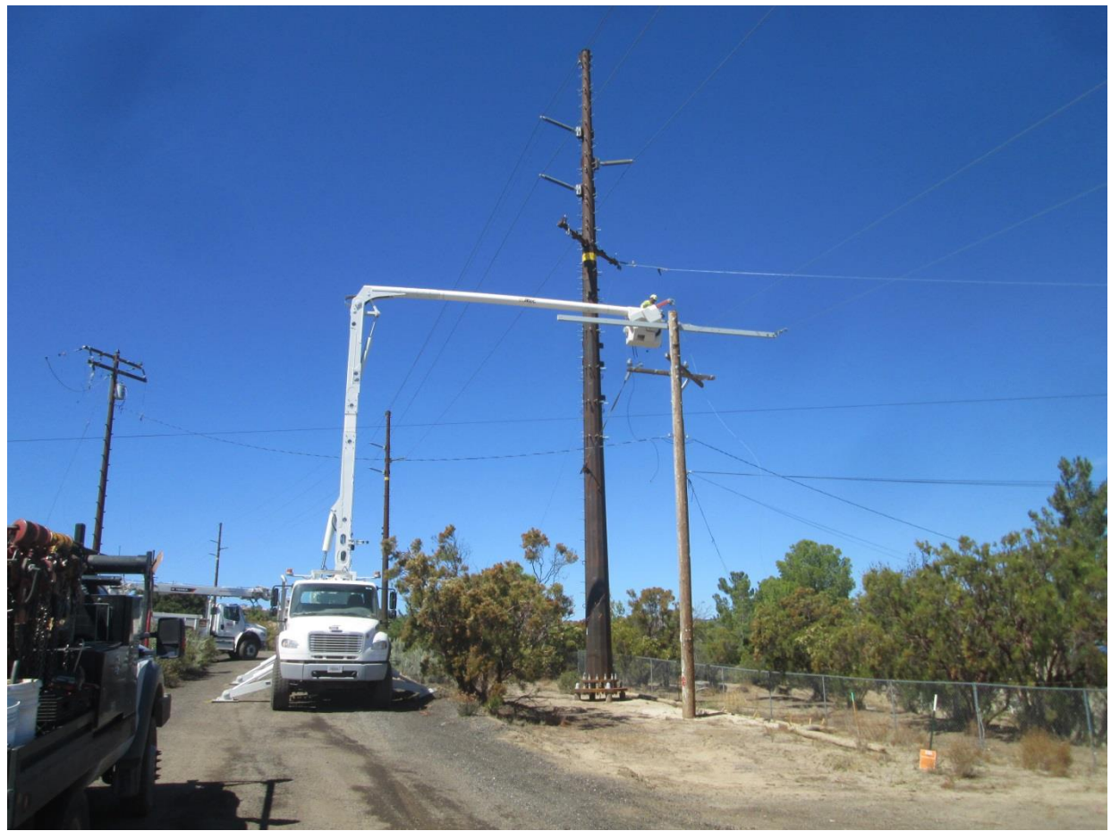
Photo 1: A construction crew observed conducting overhead line work in preparation for distribution line wire stringing at Pole P45927 (TL 6931).
